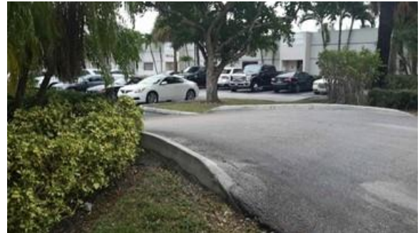
Repetitive Loss Area 9 – Building sits below grade; water runs off street toward buildings and from parking lot to building
