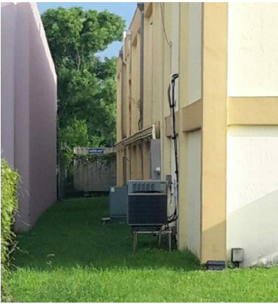
Repetitive Loss Area 6 – Elevated HVAC unit
