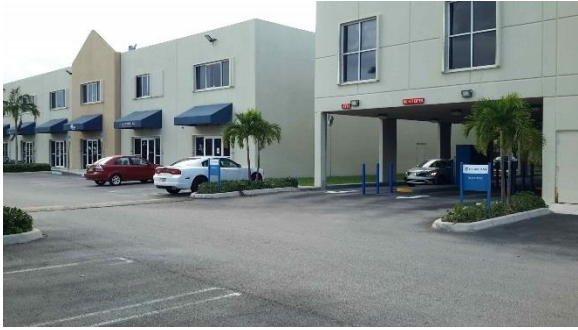
Repetitive Loss Area 21 – Parking lot slopes toward building
