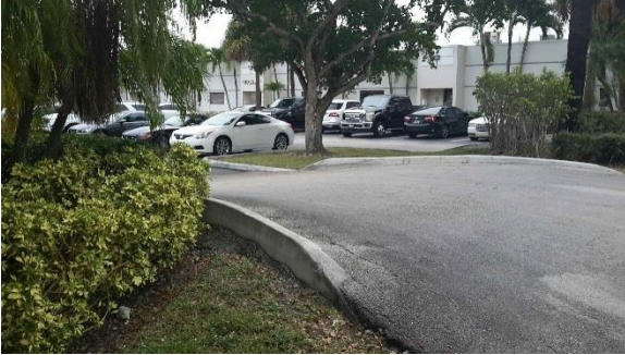
Repetitive Loss Area 11 – Building sits below grade; water runs off street toward buildings and from parking lot to building
