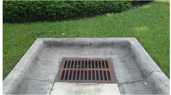
Repetitive Loss Area 2 – Drainage inlet on corner of block; curb may block entry of water
