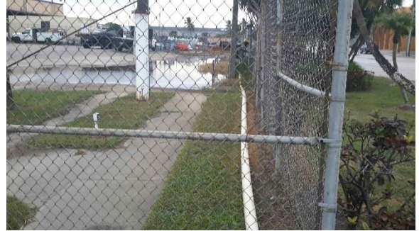
Repetitive Loss Area 12 – Pump system in place to drain parking lot
