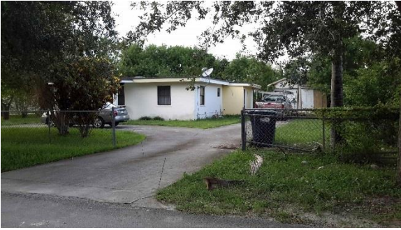
Repetitive Loss Area 20 – House below grade
