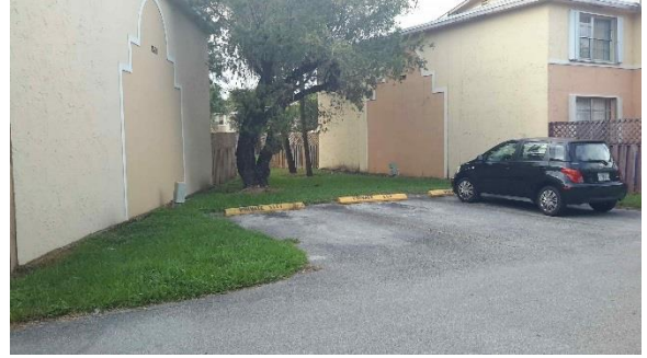
Repetitive Loss Area 10 – Buildings at grade; no guttering
