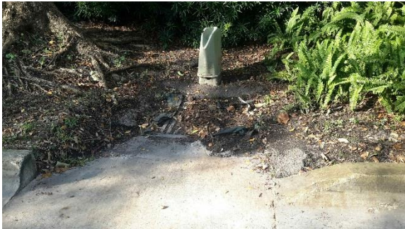
Repetitive Loss Area 3 – Clogged drainage inlet
