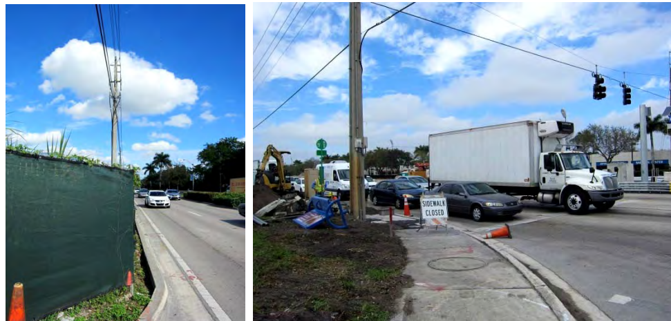
(L) Construction fence eliminates possible pedestrian pathway on NW 58 th Street. (R) Though the sidewalk is closed, the expanse of the construction makes it difficult to determine an appropriate detour route. The lack of a crosswalk also complicates matters here on NW 25 th Street.
