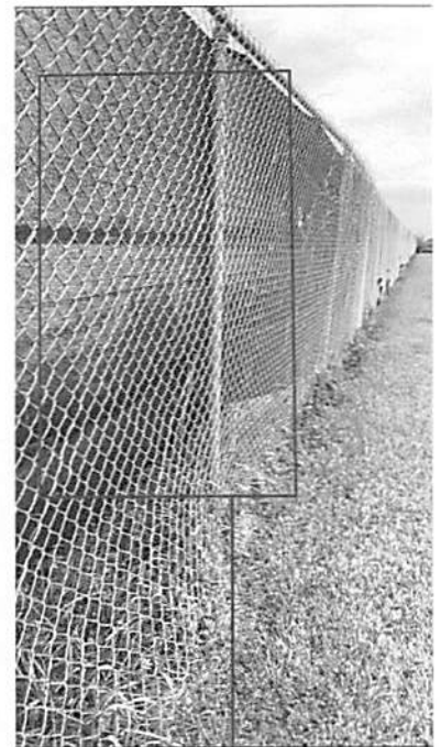
Fencing which is removed at North Property line to be replaced to match existing
