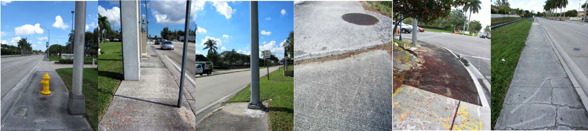
Issues encountered during a Field Analysis included (From Left to Right): Non-ADA compliant sidewalks, infrastructure obstacle course, missing sidewalks, uneven sidewalks, post maintenance issues, cracked sidewalks
