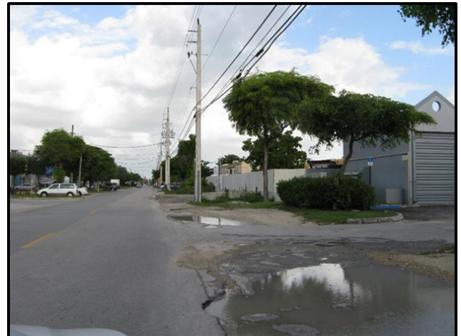
Figure IV-22 Downtown Doral – Adaptive Reuse Area – Lack of Curb and Sidewalk
