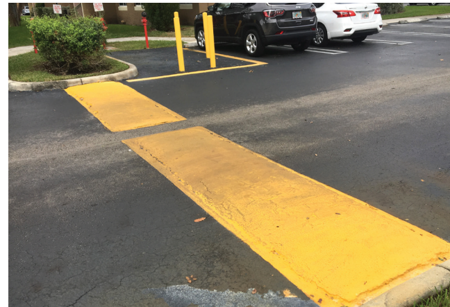
FIGURE 26. Speed bumps pavement markings
