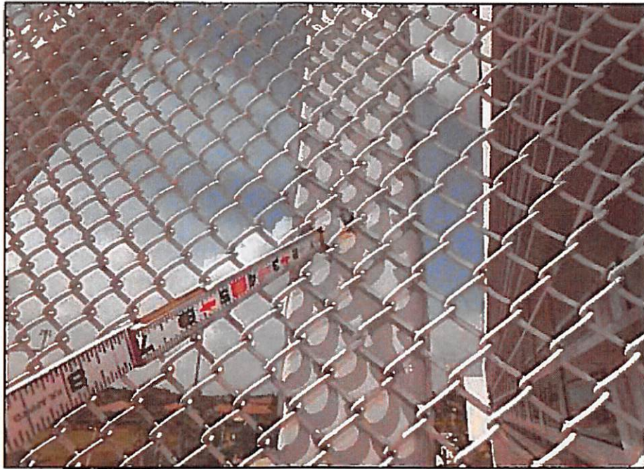
Photo 03: Typical missing connection fastener to vertical truss member on the chain-link fence. (Shown Vertical member # 2)
