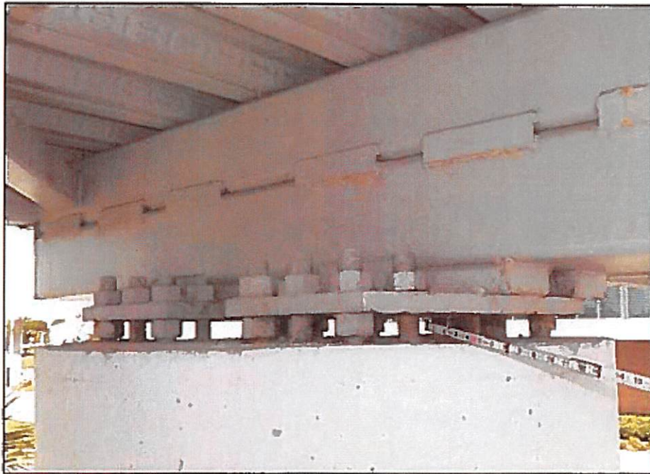
Photo 07: Only 8 out of 24 leveling nuts are installed at the fixed bearing above the east column. There is light surface corrosion on the anchorage hardware and bearing plates.
