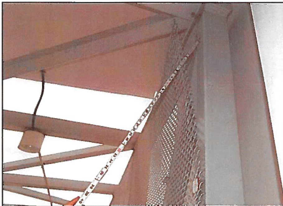
Photo 02: Missing fastener at the west end, top corner of the chain-link fence.
