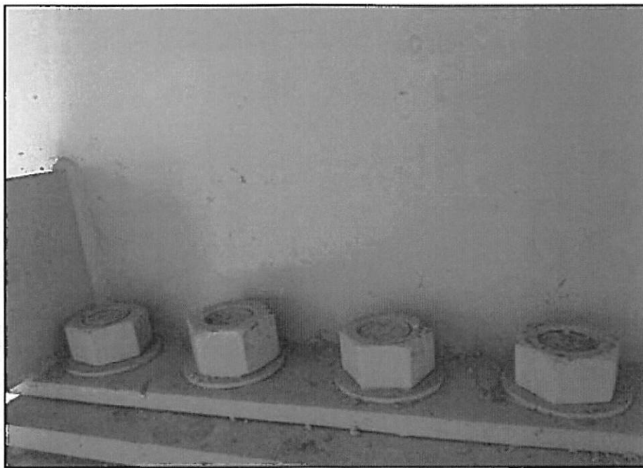
Photo 06: Typical view of the anchor bolt nuts engagement at east face of the slide bearing.
