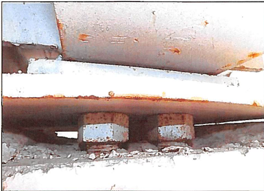
Photo 08: Light surface corrosion on the anchorage hardware and bearing plates at the slide bearing above the west column.
